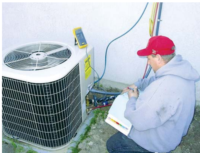
This technician is taking the final readings for a third-party verification of a high-quality installation.
