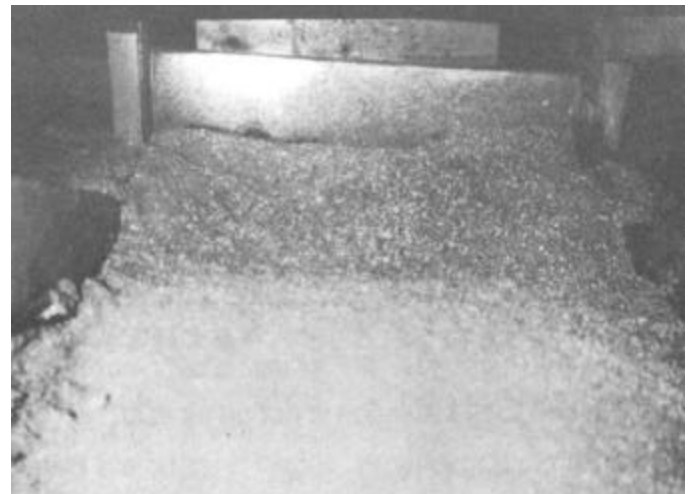
Figure 4 – Attic insulated with cellulose. Settling over soffit was caused by insulation being wetted by moist air leakage through attic floor.
