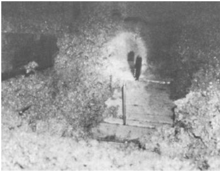
Figure 5 – Attic floor showing points of air leakage.
