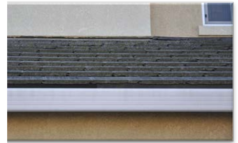
Outdated roof systems
