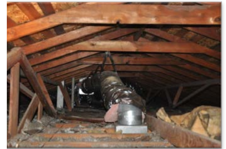
Minimal ceiling insulation, no wall or raised floor insulation, poor duct system in attic
